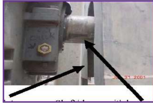
Slot opening is too large. Shaft/shelve with key way is not sufficiently guarded.
